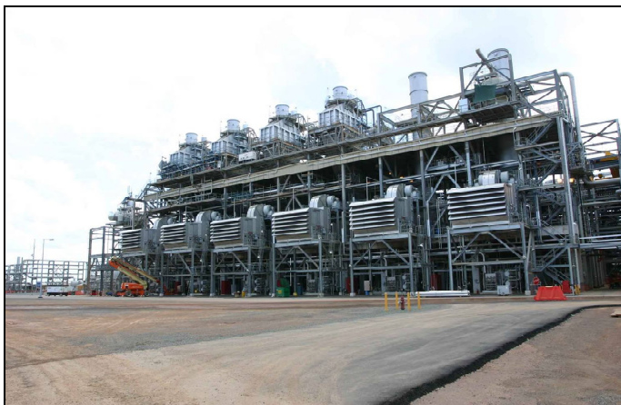
Figure 4. Photograph of compressor trains at Darwin LNG. View of the inlet filter ducts and once through steam generators (heat recovery units) on four gas turbines on the left.
